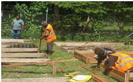
NHBG workers constructing nursery beds and arranging of plants in nursery beds
